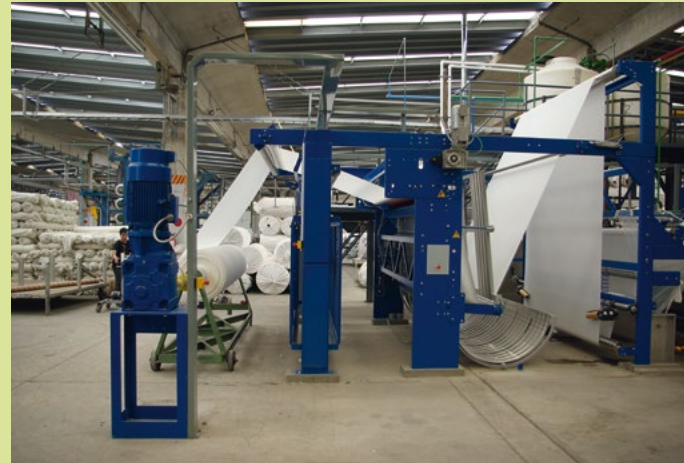
Entry area of a Pad-Dry-Bake unit
