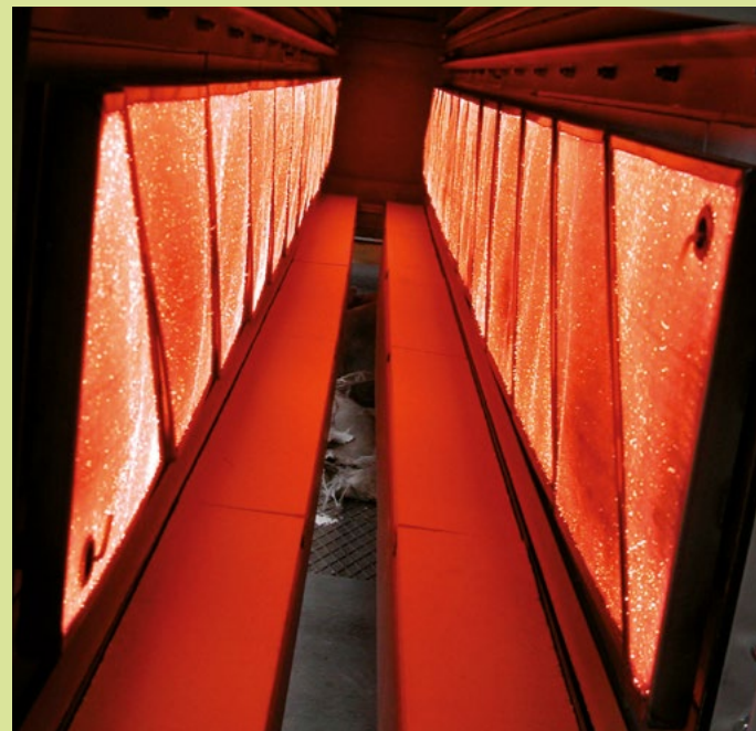
Burner elements in operation
